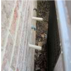
T&P drains too close
