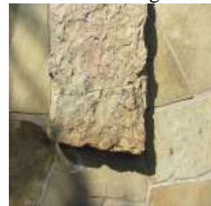
Decorative rock cracked
