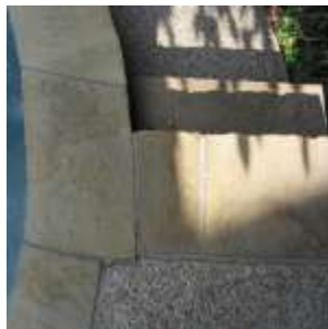
Deck & coping separation
