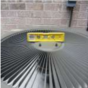
Condensing unit not level
