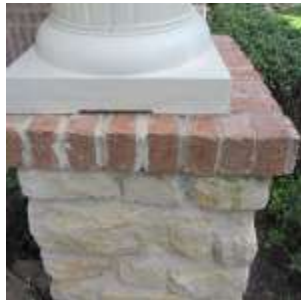
Minor brick separation
