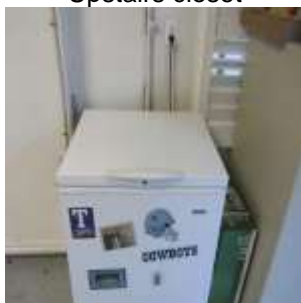
Freezer plugged into GFCI
