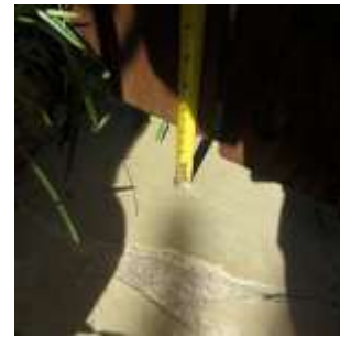
Gate too high
