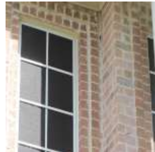
Minor brick separation
