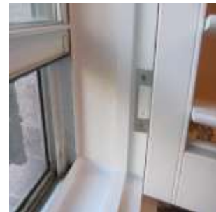
Prior water intrusion
