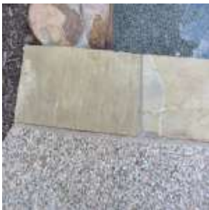
Deck & coping separation
