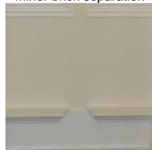
Prior wall damage
