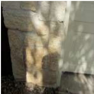
Minor brick separation
