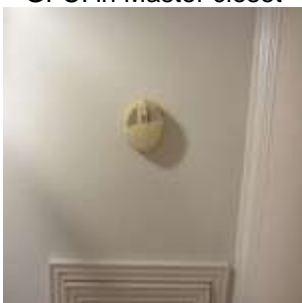
Upstairs smoke detector
