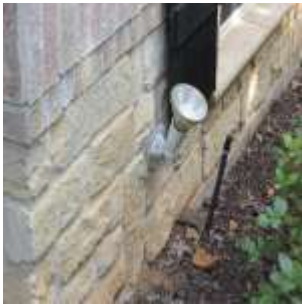
Exterior light water protection
