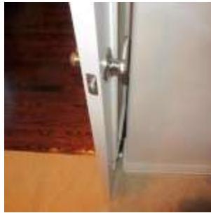
Missing door stop
