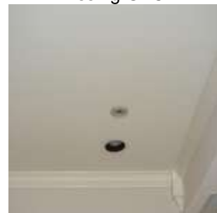
Missing smoke detector
