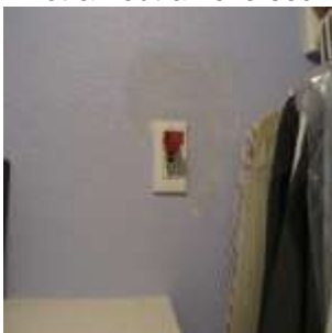
GFCI in Master closet
