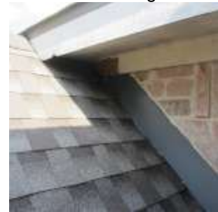
Pest damage to fascia
